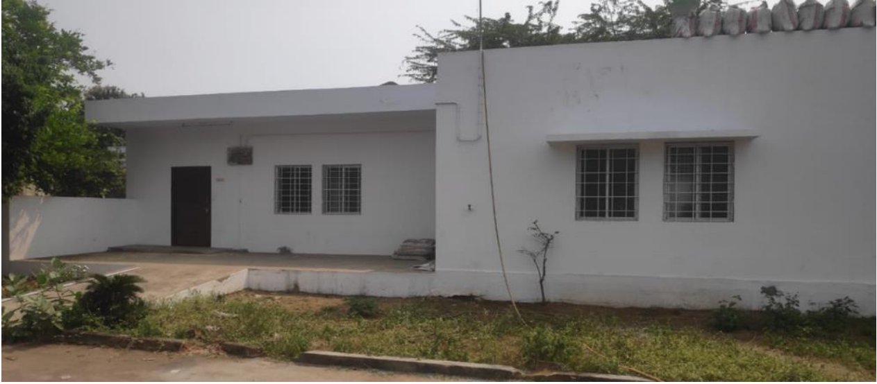
Renovation work carried out in the Dispensary at Siddha Raja Kandigai village
